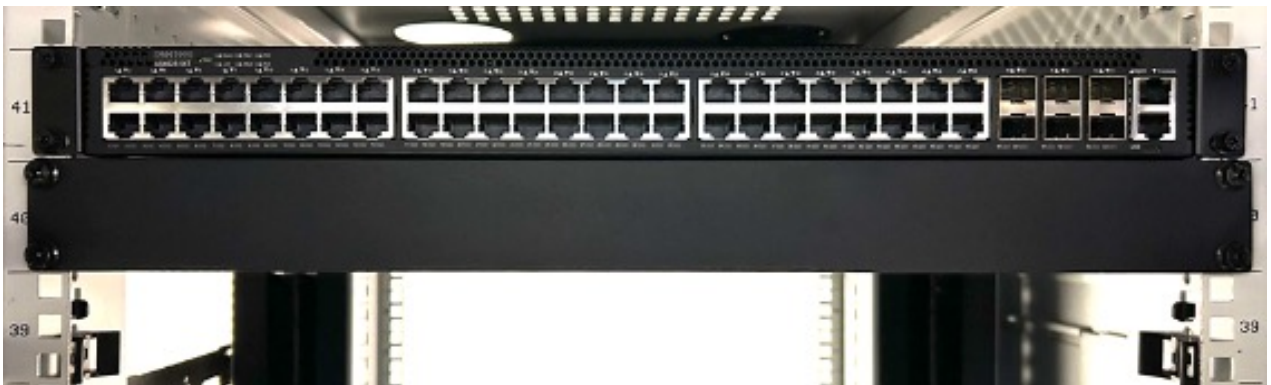
Figure 130. View from the switch ports side: Example of a properly installed MTM 5149-N64 switch and airflow control shelf
